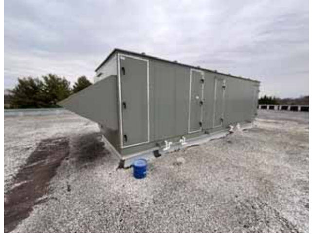
20 - ROOFTOP PACKAGED UNIT
